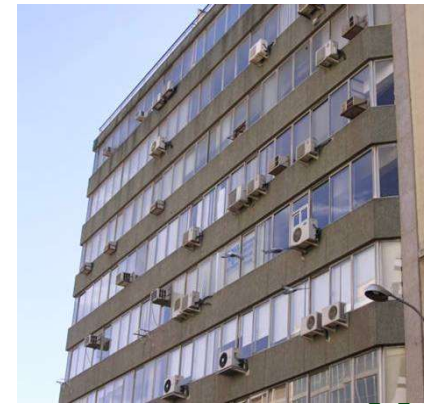
Poor Air Conditioning systems trying to mitigate the consequences of deficient Building skins
